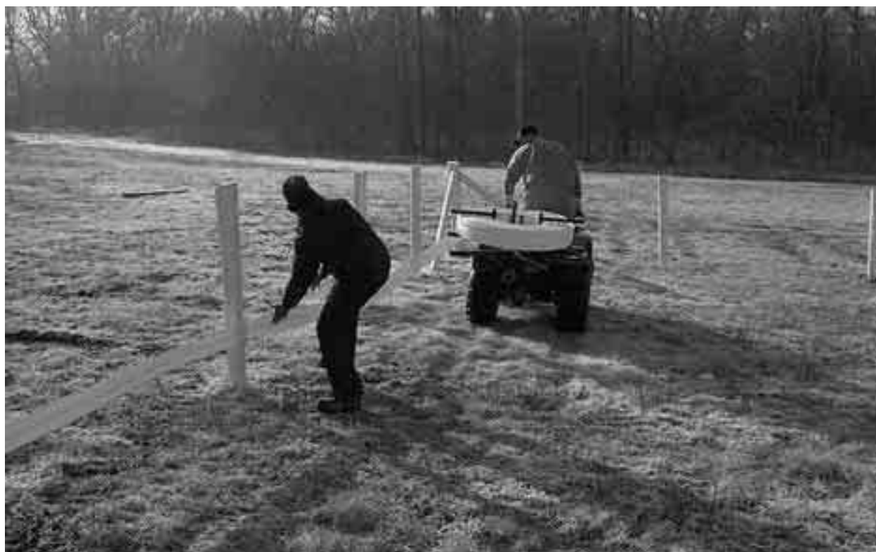
Photo 6-7. Paying out the rail with a spinning jenny mounted on the back of a 4-Wheeler.
